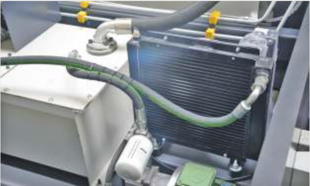
Hydraulic Oil Cooling System
